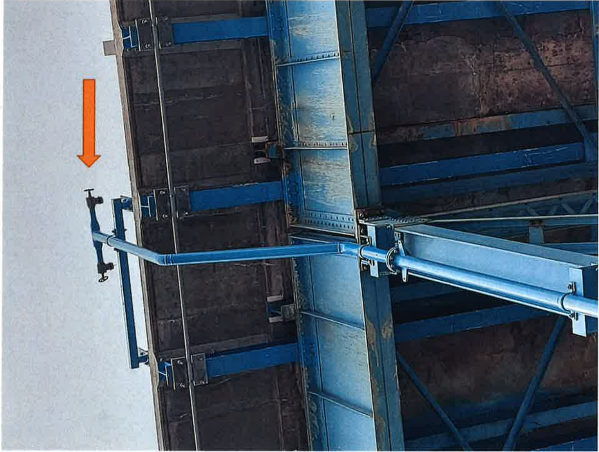
The top of the riser has two 2 ½ inch connections with a gate.
